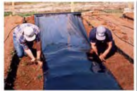
Burying the edges of plastic mulch in pathways using the trench method.
