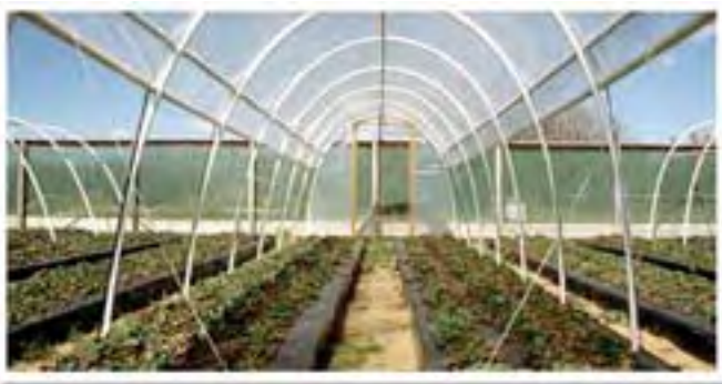
10-foot-wide moveable hoop house constructed of 1-inch diameter PVC pipe and cabling for added strength
